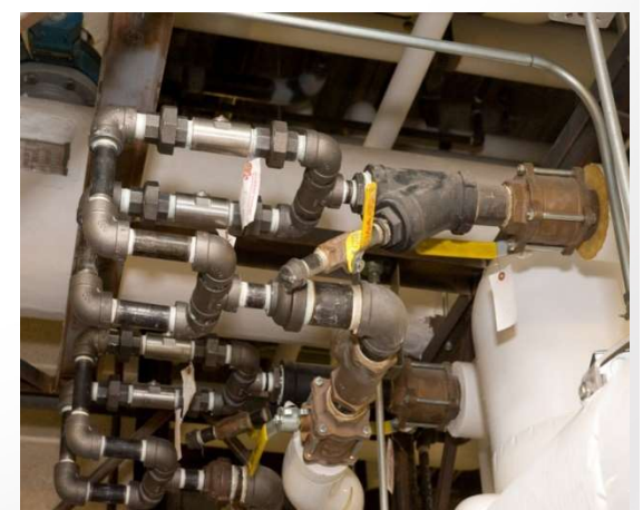
Insulation & steam traps
